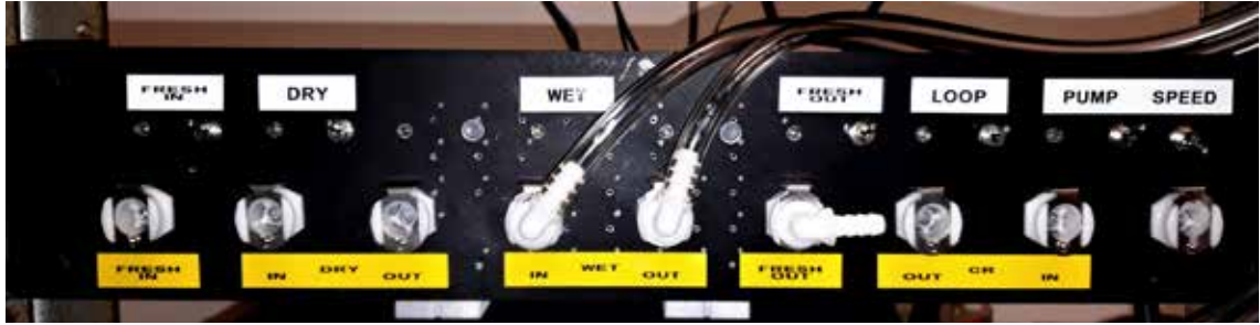
Fig. 3I Hydraulic connections and manual switches.
